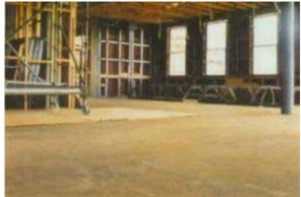
and in institutional building such as the gym at Tuggeranong College in Canberra
